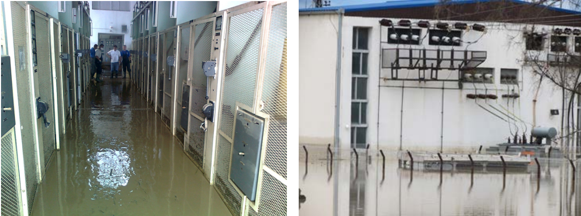
Figure 2 - Flooded substation at Orasje (left) and Doboј (right)
