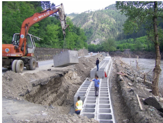
Figure 7 - Eroded segment of M-17 north of Maglaj under repaired
