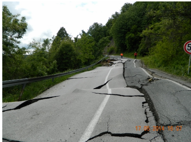
Figure 5 - Landslide destroyed regional road near Tuzla
