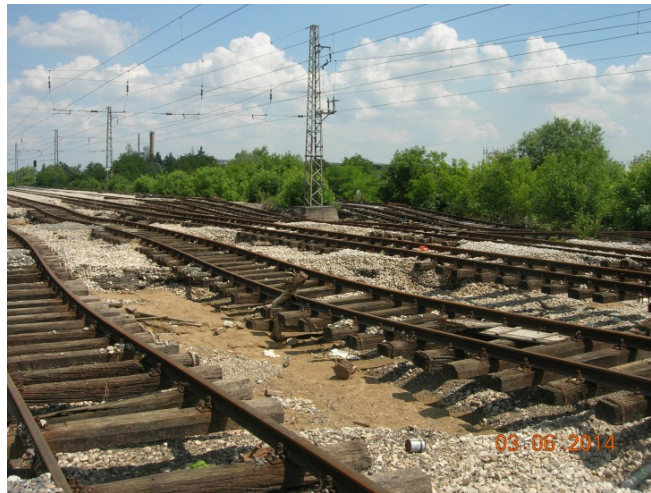
Figure 8 - Samac railway station complete wash out of ballast
