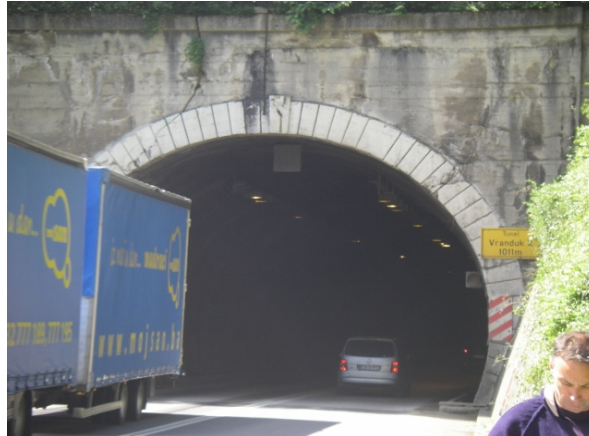
Figure 12 - Vranduk tunnel portal with visible cracks
