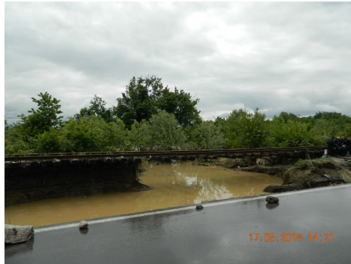
Figure 9 - Railway ballast and road embankment wash out
