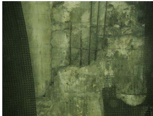
Figure 13 - Vranduk tunnel corroded reinforcement bars of the final lining
