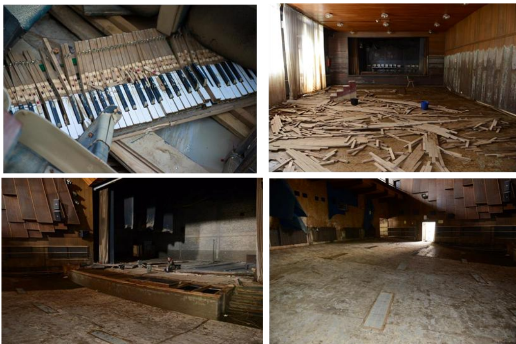
Figure 1-34. Cultural center of Obrenovac. The situation after the withdrawal of water. The picture top right shows the small theater hall, the line of flooded level is evident. The two pictures bottom right and left show the great theater hall after the remove of parterre seats and the damage to the revolving rotation system of the theater stage. events and sport activities) is lost for all the time of closure. The local city summer festival,
